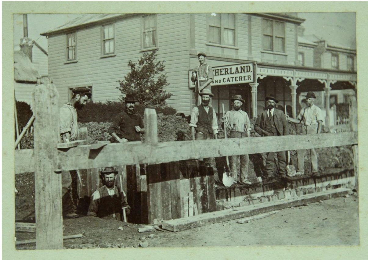
Christchurch Drainage Board: Sewer construction east end of Tuam St c1905 Source: CH659/100 – 10/208470
